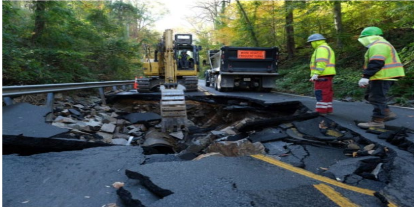
13. Sinkhole caused by large water main break (staff photo by Jay Westcott)
